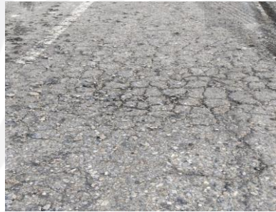
Distressed Existing Surface
