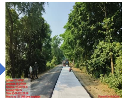
Laying of Paving fabric and Providing BC / PQC over the stabilized Layer
