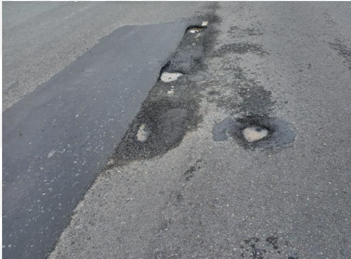
Series of Potholes
