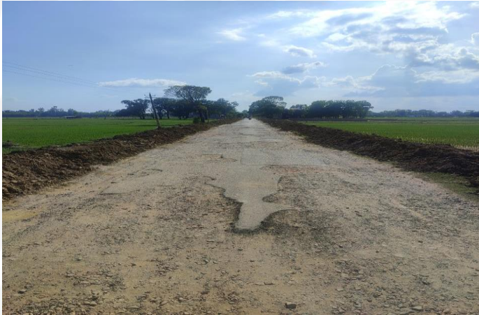
Highly Distressed/Base or Subbase Failure
