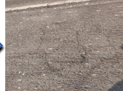
Cracked Surface after Milling up to required thickness
